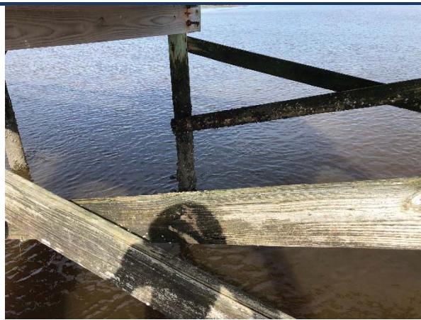
Photo 1: Missing lateral bracing at the fishing pier terminus platform
