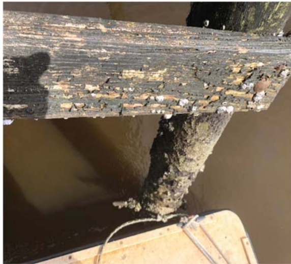
Photo 2: Rusted fasteners and heavily weathered lateral bracing at the fishing pier terminus platform
