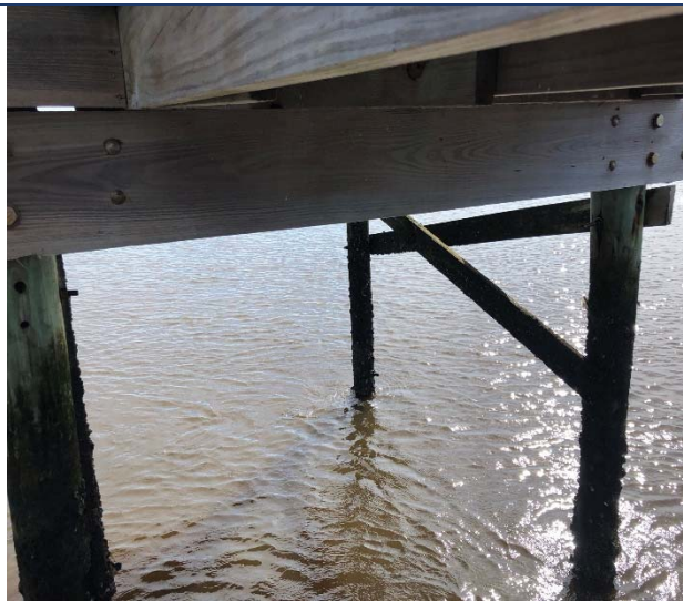
Photo 6: Missing lateral bracing at the fishing pier terminus platform
