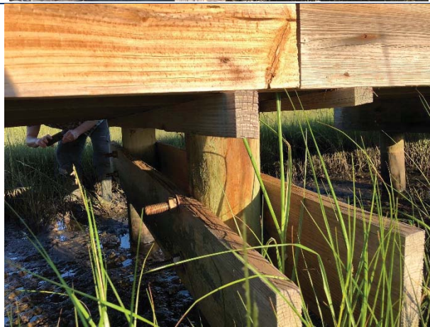
Photo 4: Damaged girders. Boardwalk joist and deck framing completely separated from girders and piles.
