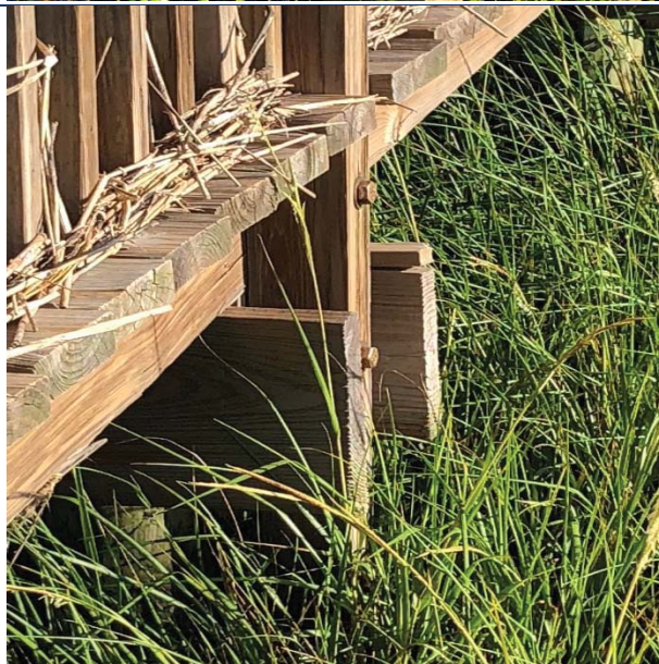
Photo 5: Damaged girders at beginning of bridge ramp up
