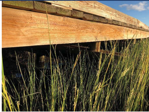
Photo 1: Boardwalk separated from the piles and girders
