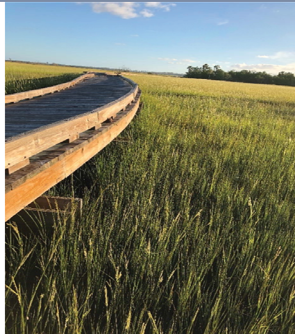
Photo 2: Displacement of boardwalk deck and joists.
