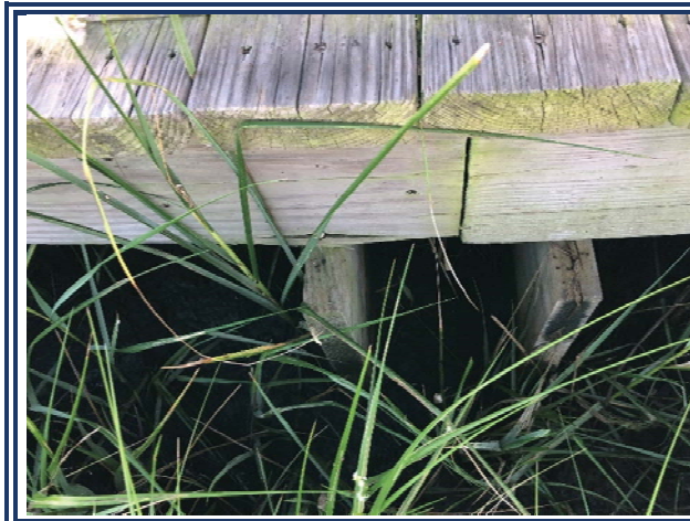
Photo 6: Damaged deck joist connection. The screw had begun to pull through the deck joist.
