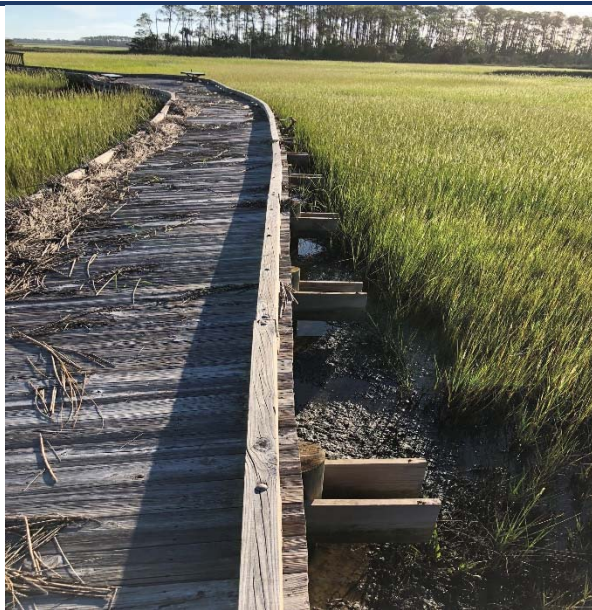
Photo 3: Displacement of boardwalk deck and joists.
